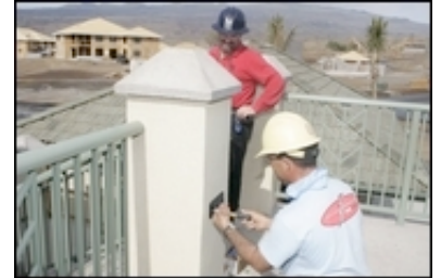
Anthony Perry, right, and Travis Tjarks, both of Kona, work on a house in the resort subdivision of Wai'ula'ula at Mauna Kea Resort on the Big Island. Residences in this Kohala Coast resort range from about $1 million to $3.5 million. Resort home sales soared last year.
